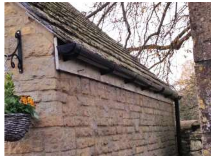
'facia boards should not be used for fixing gutters'
